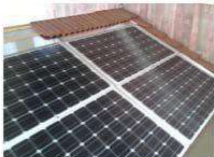
Installation photovoltaïque raccordée
